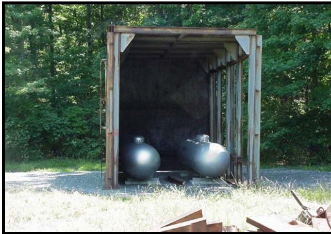
Figure 7. Shielded Propane Fuel Tanks.
