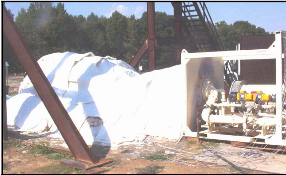
Figure 1. Transportable Hot Gas Decontamination System and Insulation Blanket.
