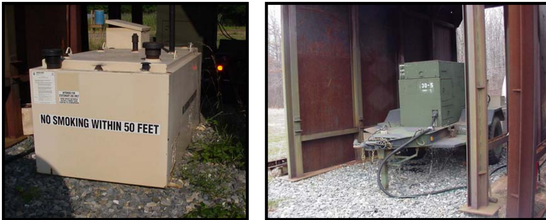
Figure 3. Shielded Diesel-Powered Generator and 500-Gallon Auxiliary Tank.
