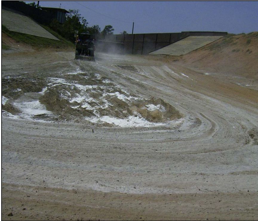
Figure 10. Using a cultivator and rake to mix the lime into the Fort Jackson HGR soil to a depth of approximately 6 in
