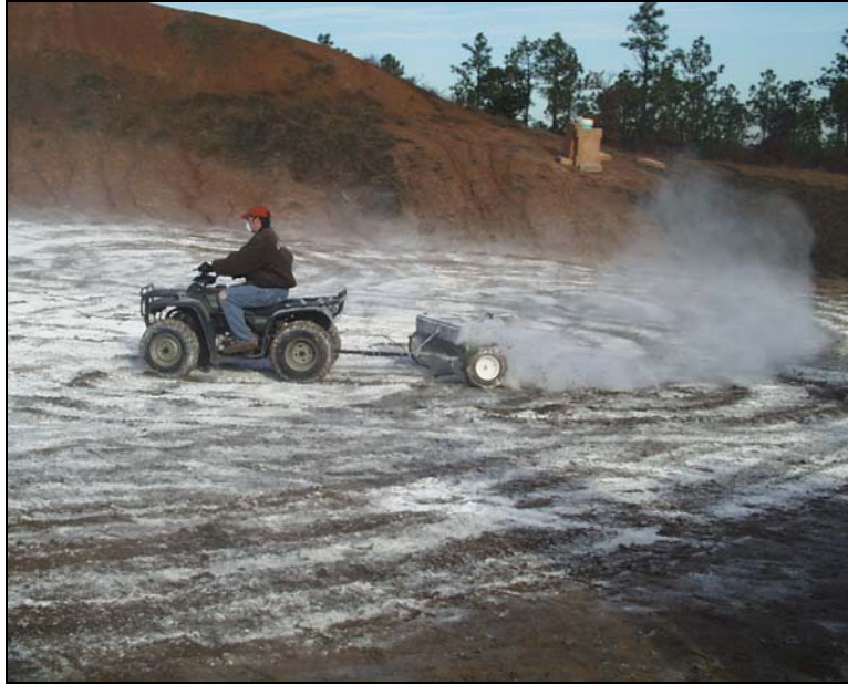
Figure 16. Using an ATV and the drop spreader to apply the lime to top of the HGR soil
