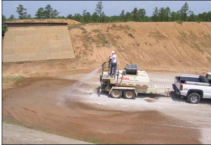
Figure 8. A hydro-seeder was used after the final lime application to evaluate its effectiveness for dust control
