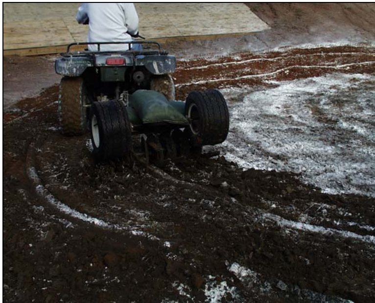
Figure 17. Using an ATV and a disc to mix the lime and HGR soil to a depth of approximately 6 in
